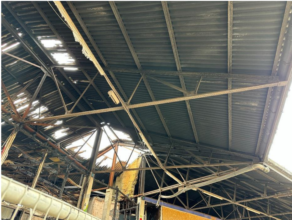
Plate 15 Main Grandstand Fire Damage
