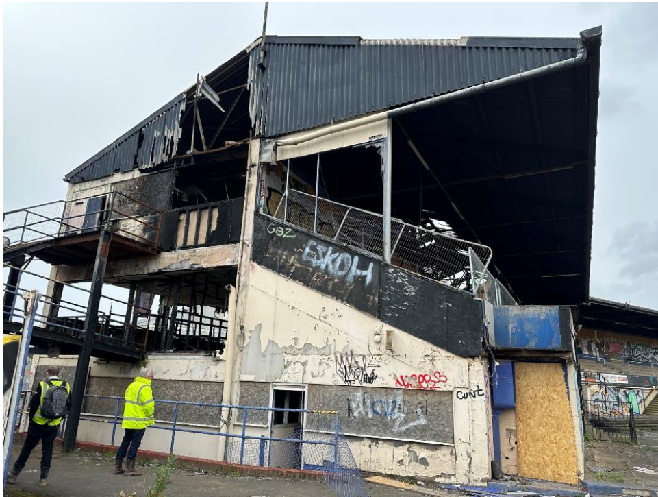
Plate 23 Main Grandstand southern end Fire Damage
