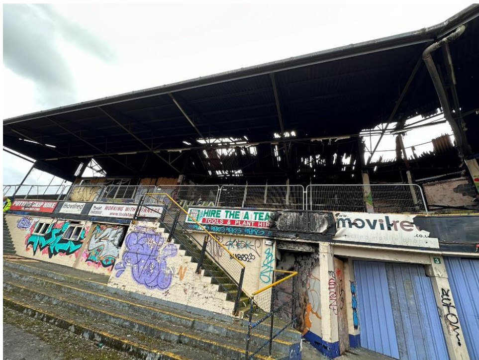
Plate 10 Main Grandstand southern section Fire Damage
