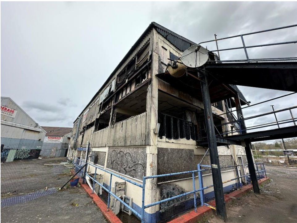
Plate 28 Main Grandstand southern end Fire Damage
