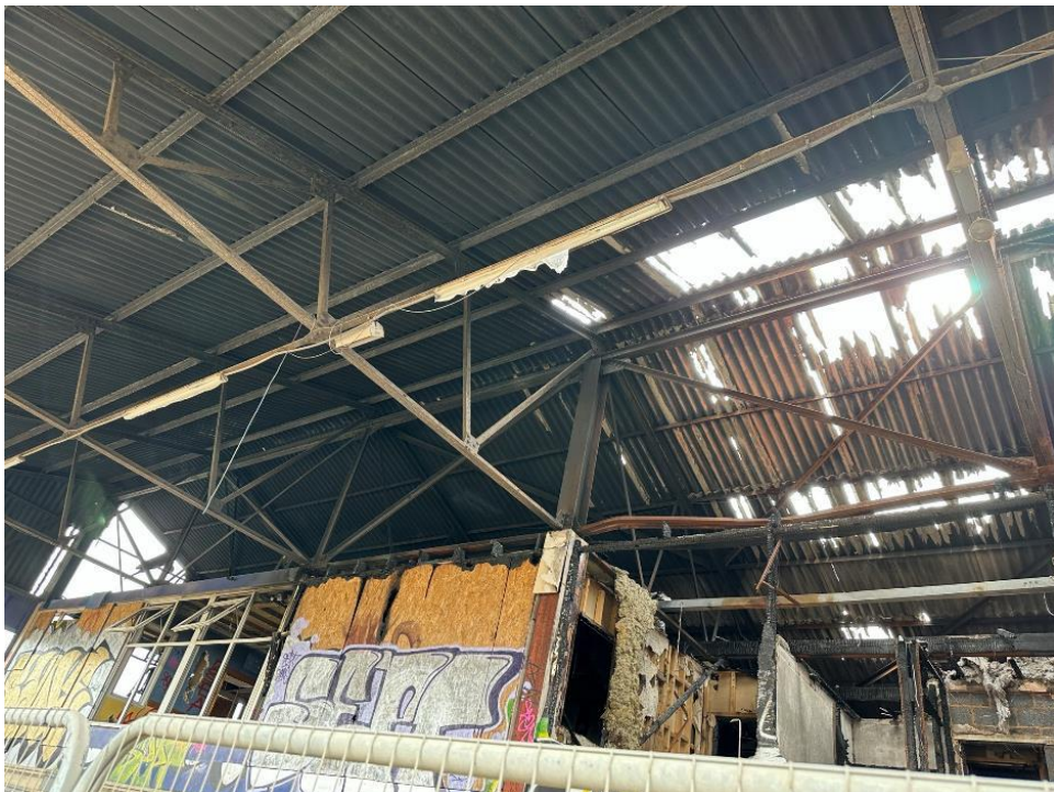
Plate 14 Main Grandstand Fire Damage
