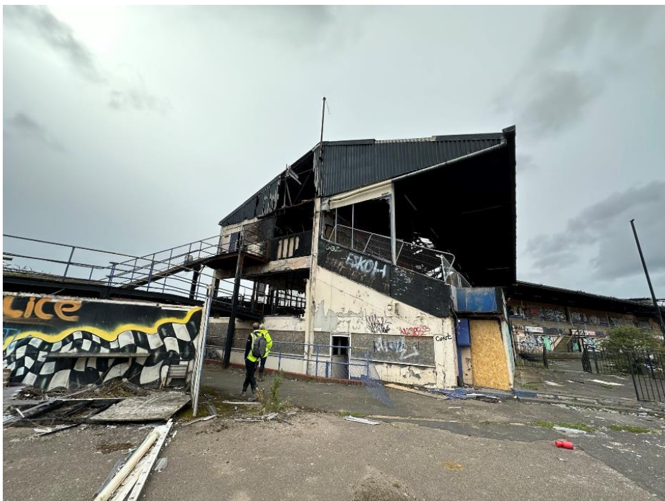
Plate 22 Main Grandstand southern end Fire Damage
