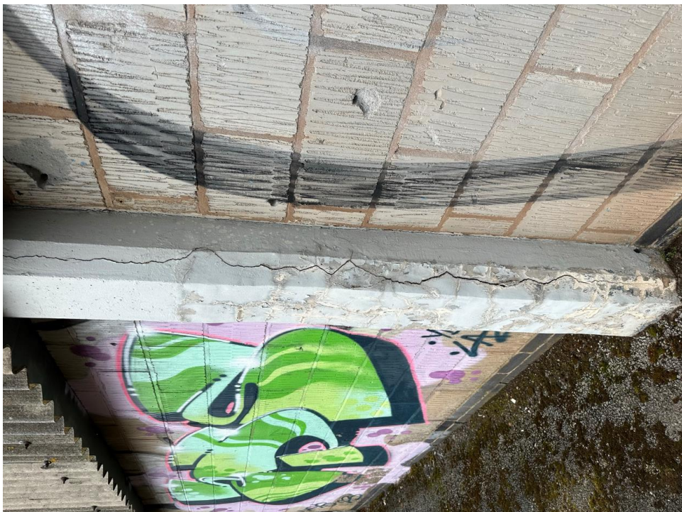
Plate 38 Main Grandstand western rear elevation cracking to column concrete
