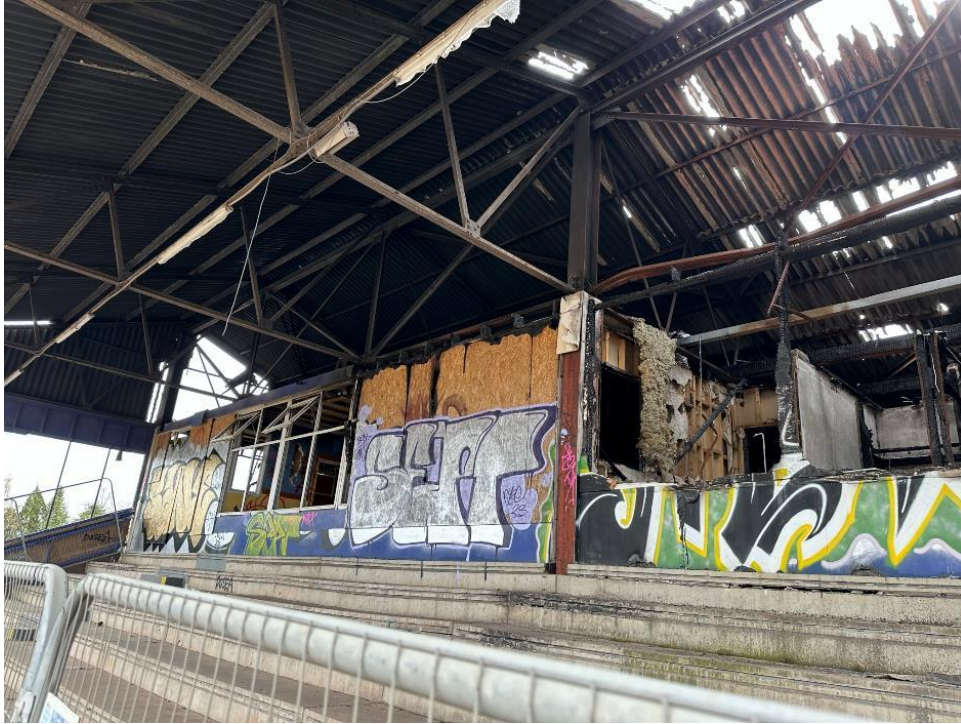
Plate 17 Min Grandstand Fire Damage
