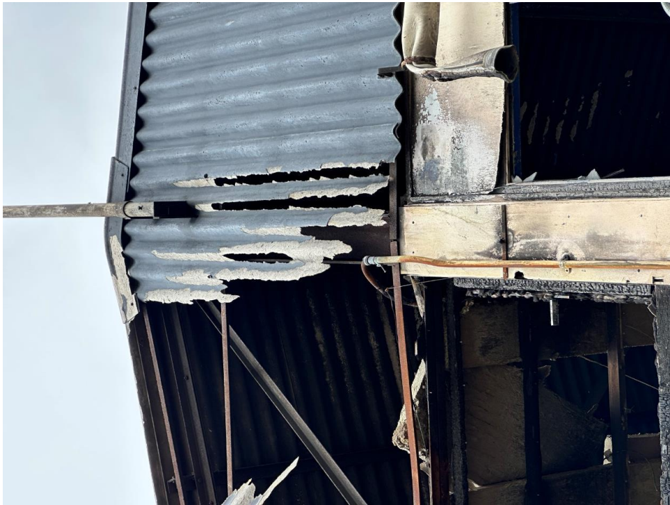
Plate 25 Main Grandstand southern end Fire Damage
