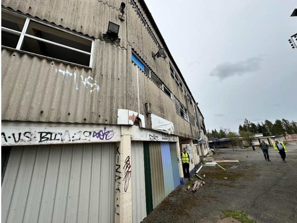
Plate 31 Main Grandstand western rear elevation Fire Damage
