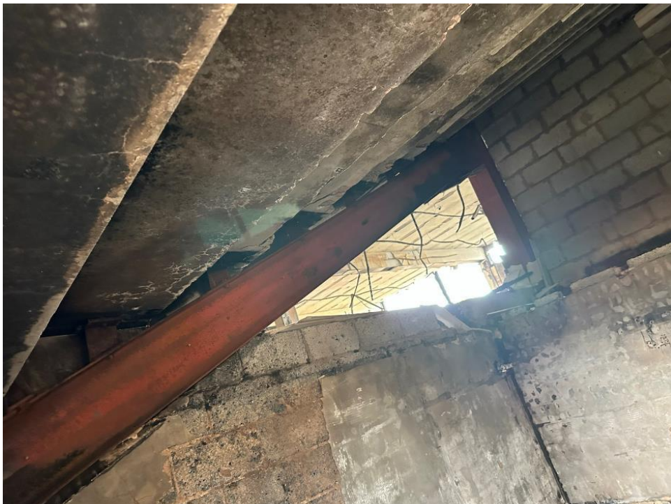
Plate 20 Main Grandstand Terrace Slab Soffit shear cracking DEFECT
