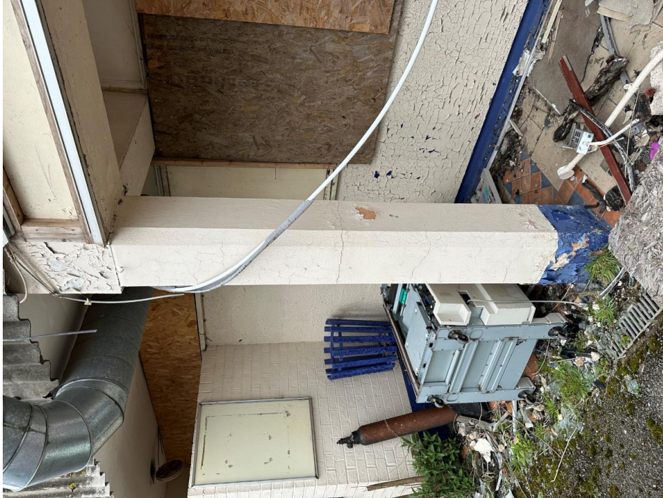
Plate 33 Main Grandstand western rear elevation cracking to column concrete
