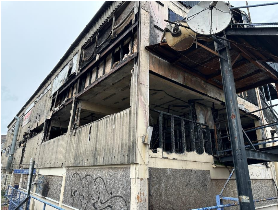
Plate 29 Main Grandstand southern end Fire Damage
