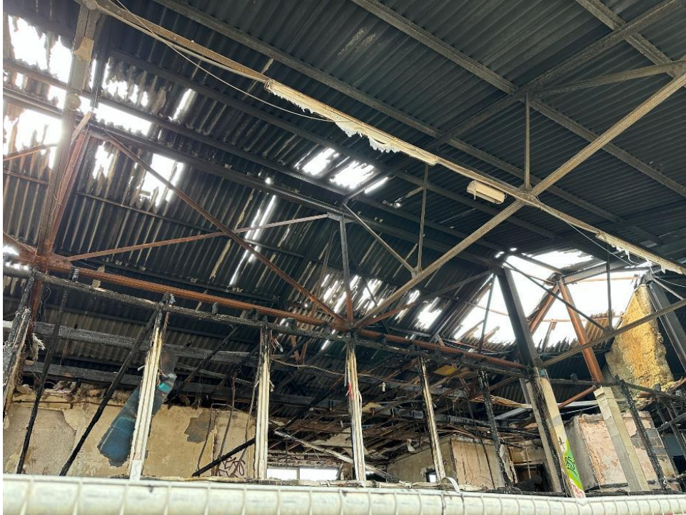
Plate 13 Main Grandstand Fire Damage
