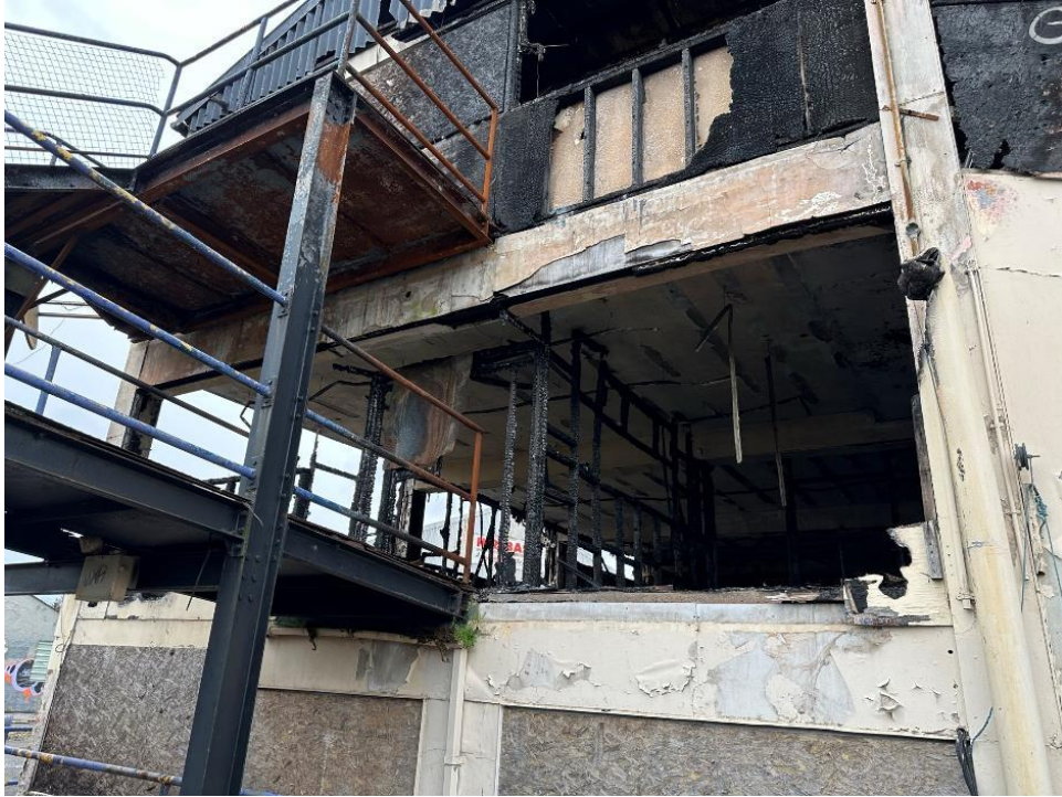
Plate 27 Main Grandstand southern end Fire Damage
