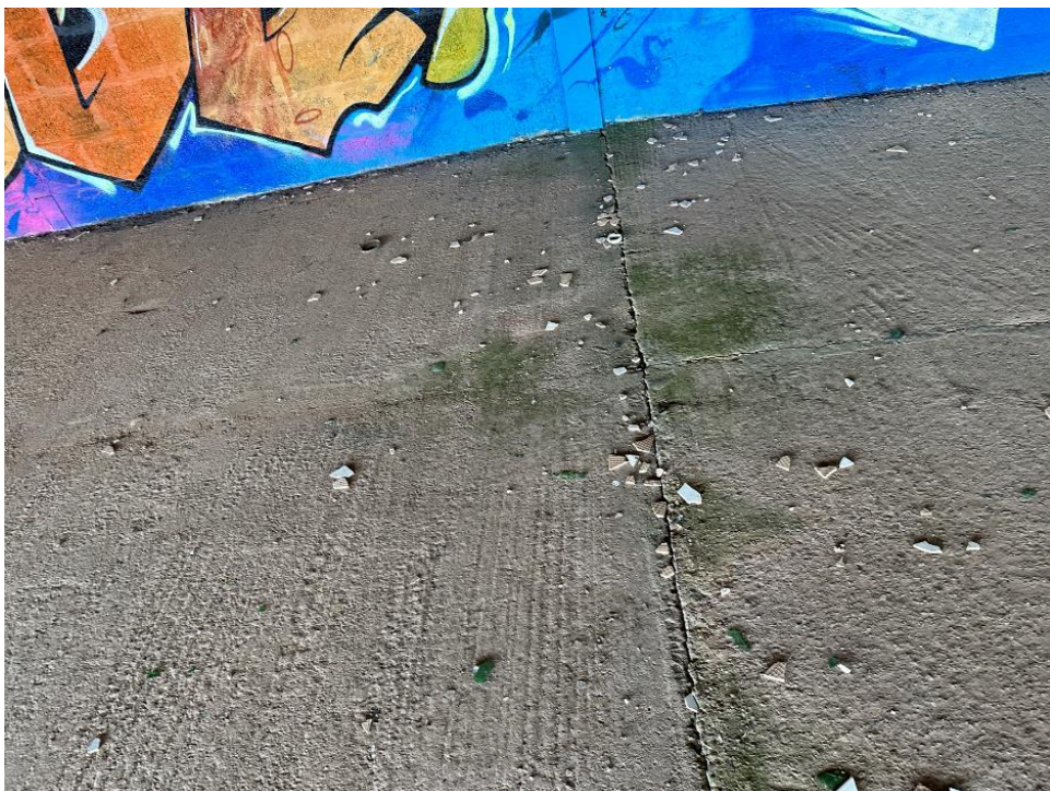
Plate 62 Eastern Grandstand terrace DEFECT
