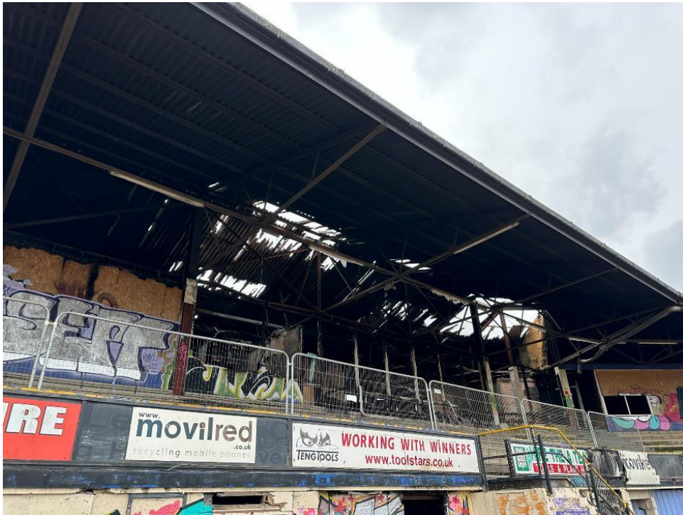
Plate 7 Main Grandstand southern section Fire Damage
