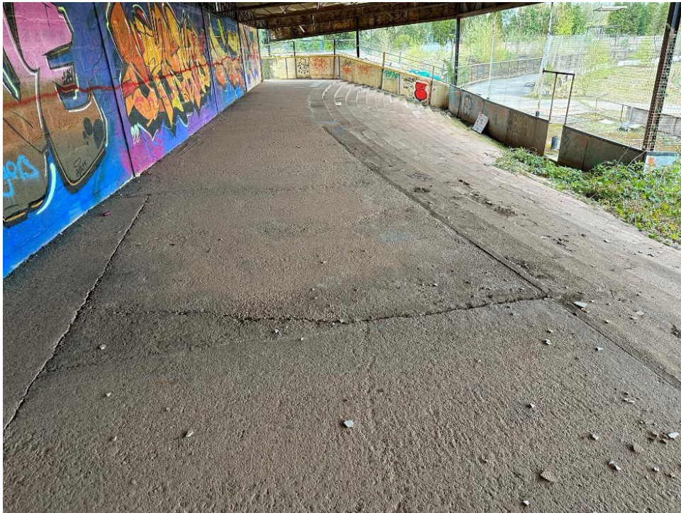
Plate 61 Eastern Grandstand terrace DEFECT
