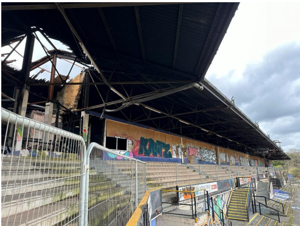
Plate 16 Main Grandstand view North Fire Damage
