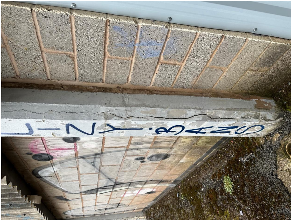
Plate 37 Main Grandstand western rear elevation cracking to column concrete
