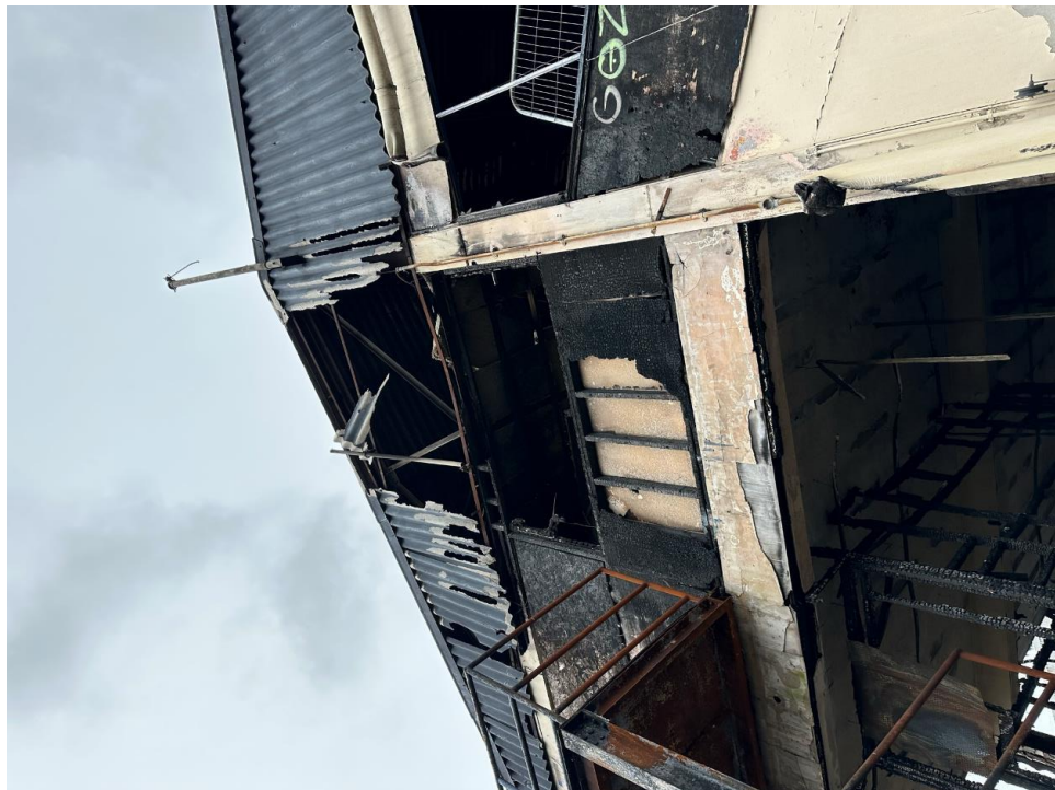
Plate 26 Main Grandstand southern end Fire Damage
