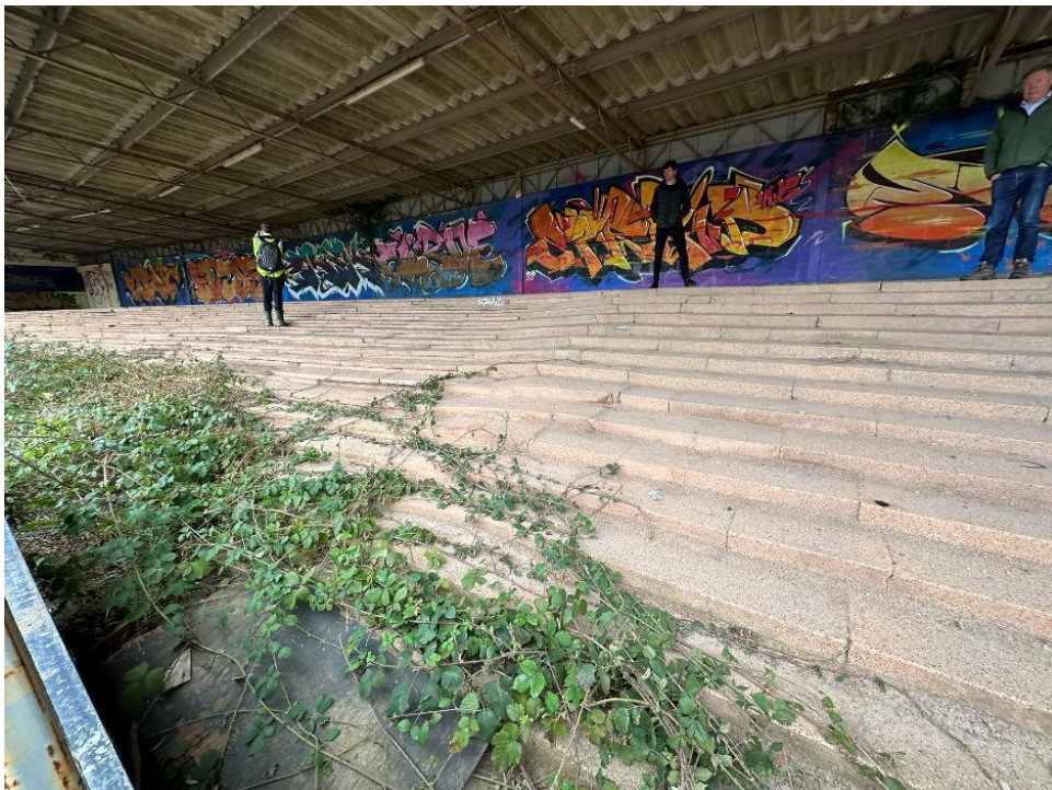
Plate 56 Eastern Grandstand southern end terrace DEFECT
