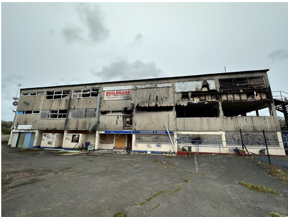
Plate 30 Main Grandstand western rear elevation Fire Damage
