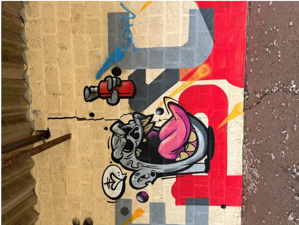
Plate 67 Eastern Grandstand rear elevation unstable wall DEFECT
