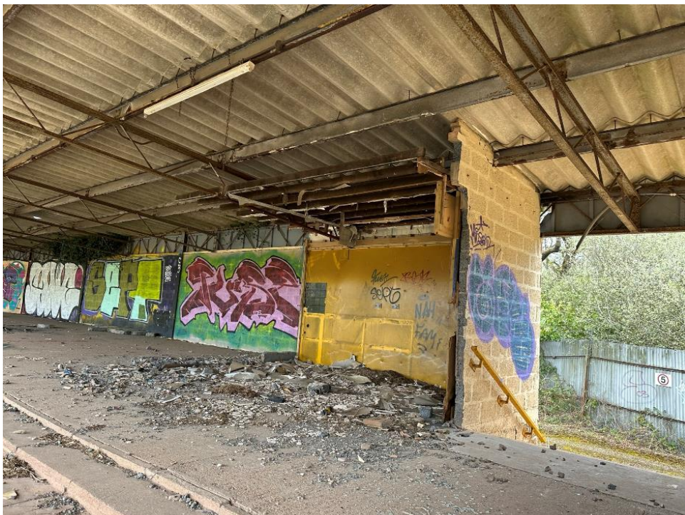
Plate 68 Eastern Grandstand rear elevation demolished toilet block unstable wall
