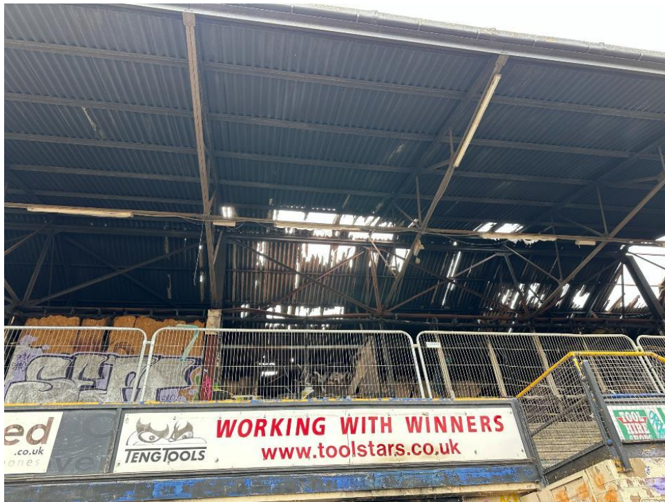
Plate 9 Main Grandstand southern section Fire Damage
