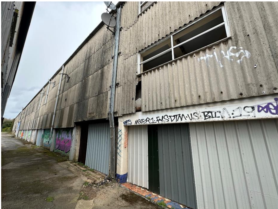
Plate 32 Main Grandstand western rear elevation Fire Damage
