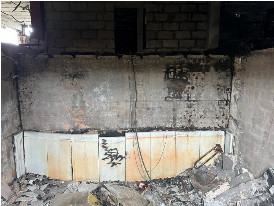
Plate 21 Main Grandstand Fire Damage to internal block walls
