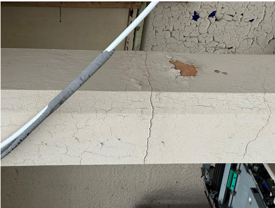
Plate 34 Main Grandstand western rear elevation cracking to column concrete
