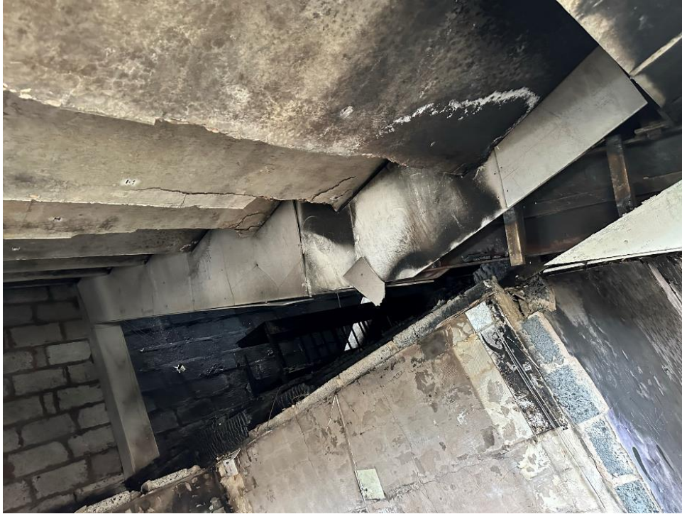
Plate 19 Main Grandstand Terrace Slab Soffit shear cracking DEFECT
