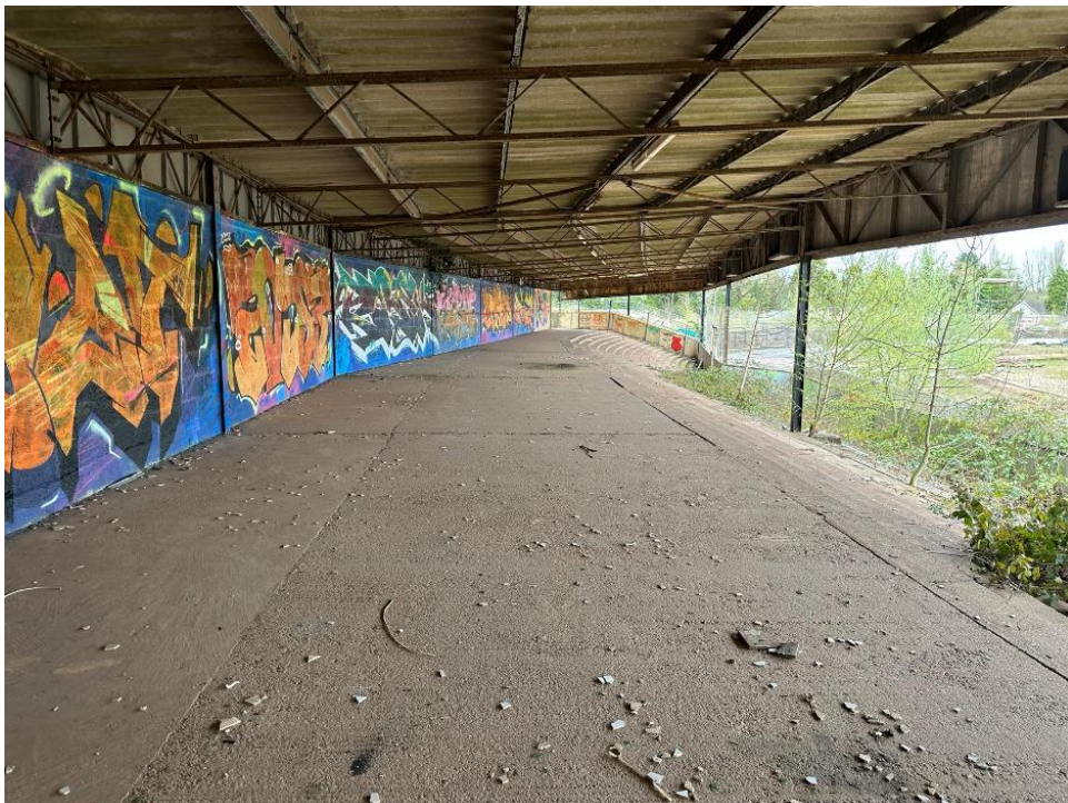
Plate 64 Eastern Grandstand terrace DEFECT
