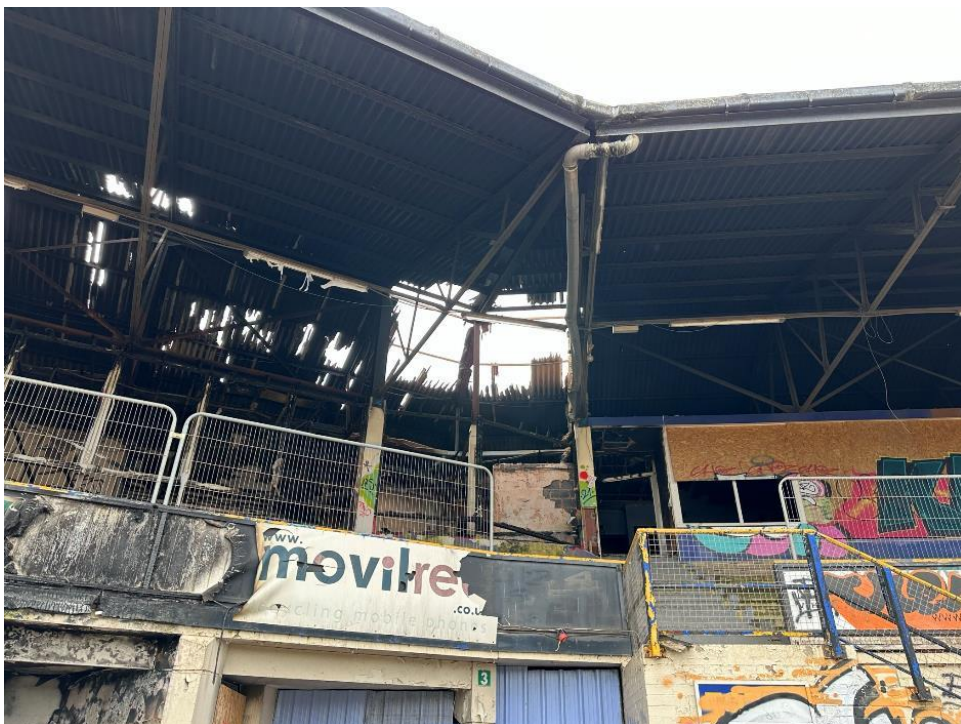
Plate 12 Main Grandstand Fire Damage
